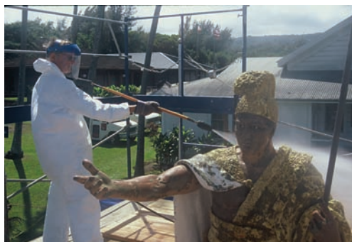
Fig. 4. Removing paint with pressurized steam blasting, one of several methods used in the process
